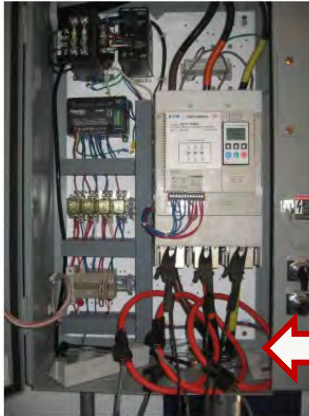
Hole 12 Well Panel Interior
